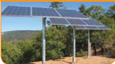
4.5 kW off-grid installation in California, USA
