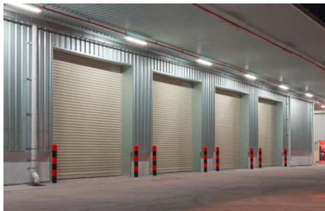
Illumination for exterior areas exposed to adverse conditions
